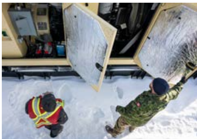
Canadian Armed Forces Technical Assessment Team member Sergeant Christopher King at work with a member of the Pimicikamak Cree Nation (Cross Lake) at a power generator in Cross Lake, Manitoba on 14 January, 2026. Photo Credit: Aviator (Avr) Daniel Bartchouk, Imagery Technician, Canadian Armed Forces Combat Camera
